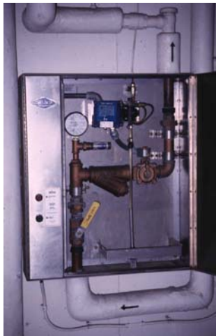
Fig. 2-10. Valve junction panel
