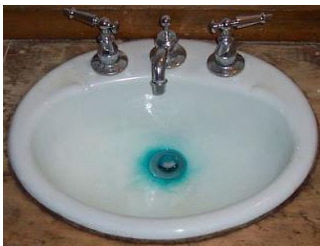
Blue-green staining caused by copper corrosion. Image from beauchampwater.blogspot.com
